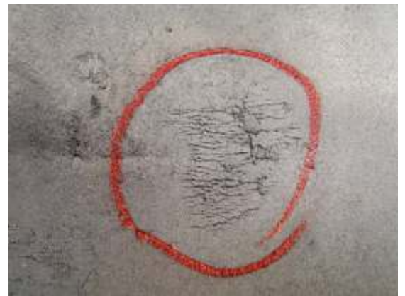
Axially oriented crack colony
